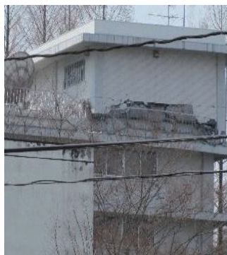
Damage of top floor of 4-story building.
