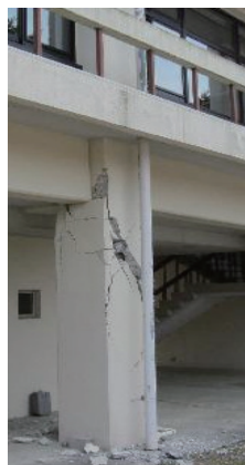
1st-floor support column in 2-story building fractured.
